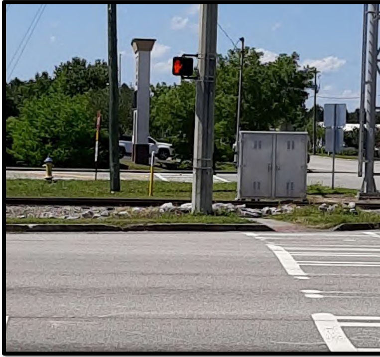
Figure 64. Pedestrian Signal Head at the Intersection Without Countdown
