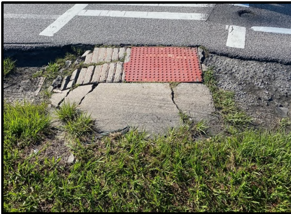
Figure 37. Damaged ADA Ramp
