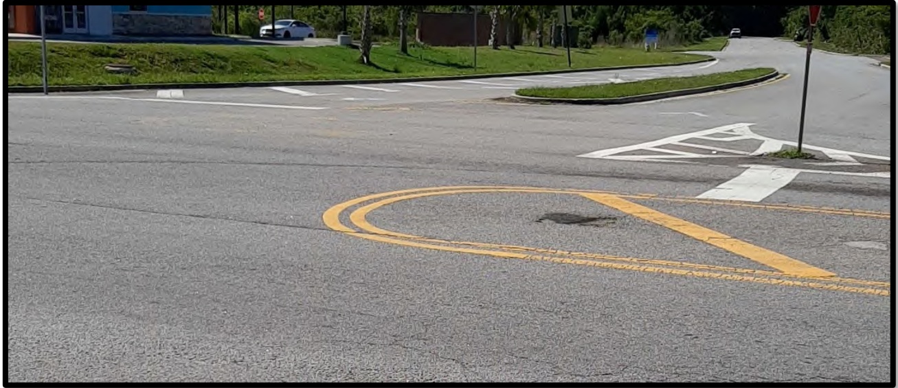
Figure 75. Fading Striping on the South Leg of the Intersection
